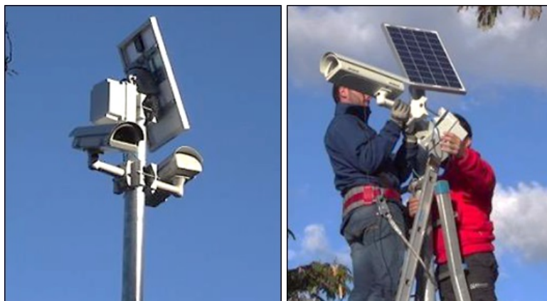
(a) Example of installation of two sensors on a single pole (b) Mounting the sensor and the photovoltaic panel on the top of the pole
